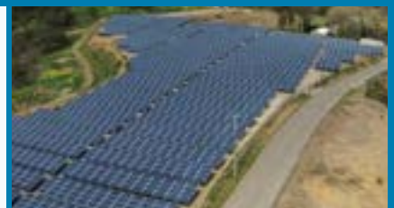
Large Scale Projects 大規模太陽能發電
